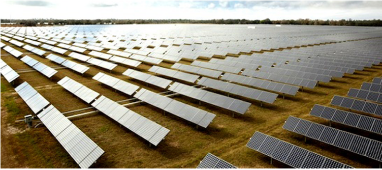
Figure 8.3 Ground-mounted PV (Source: NetZero Renewable Resources).
